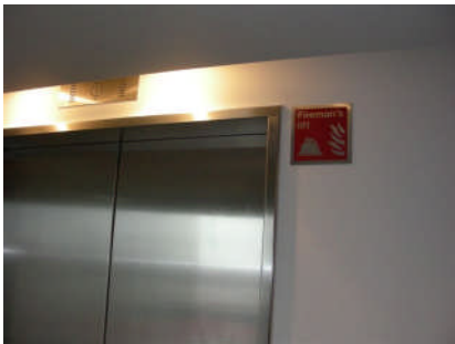
Figure 27– Fire-Fighting Lift signage
