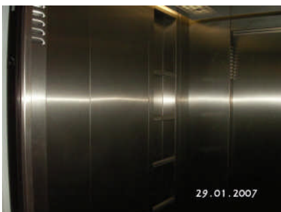
Figure 28– Fire-Fighting Lift Car
